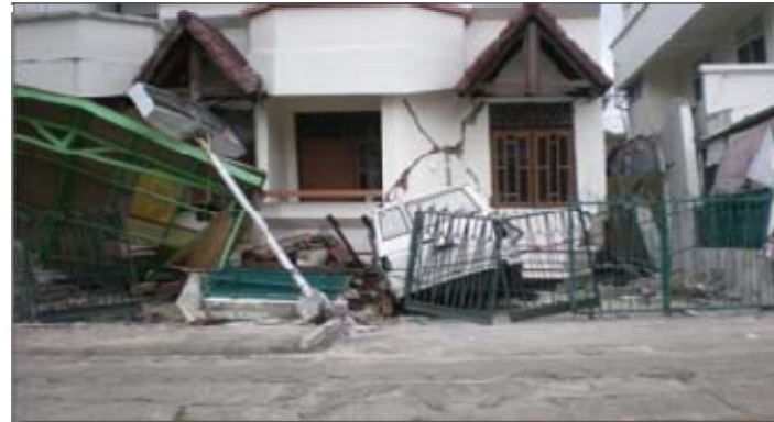
Broken houses in Padang city.
